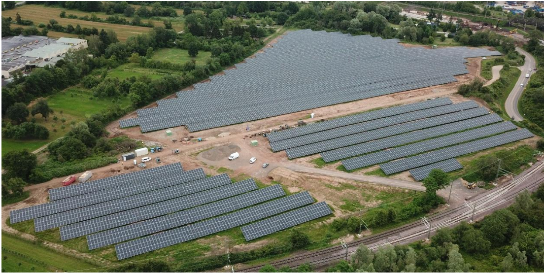
Fig.20 Trier ground power station project in Germany
